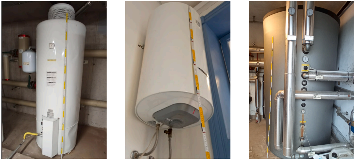
Fig. 5. DHW production (from left: gas boiler, electric boiler and solar panels storage).
