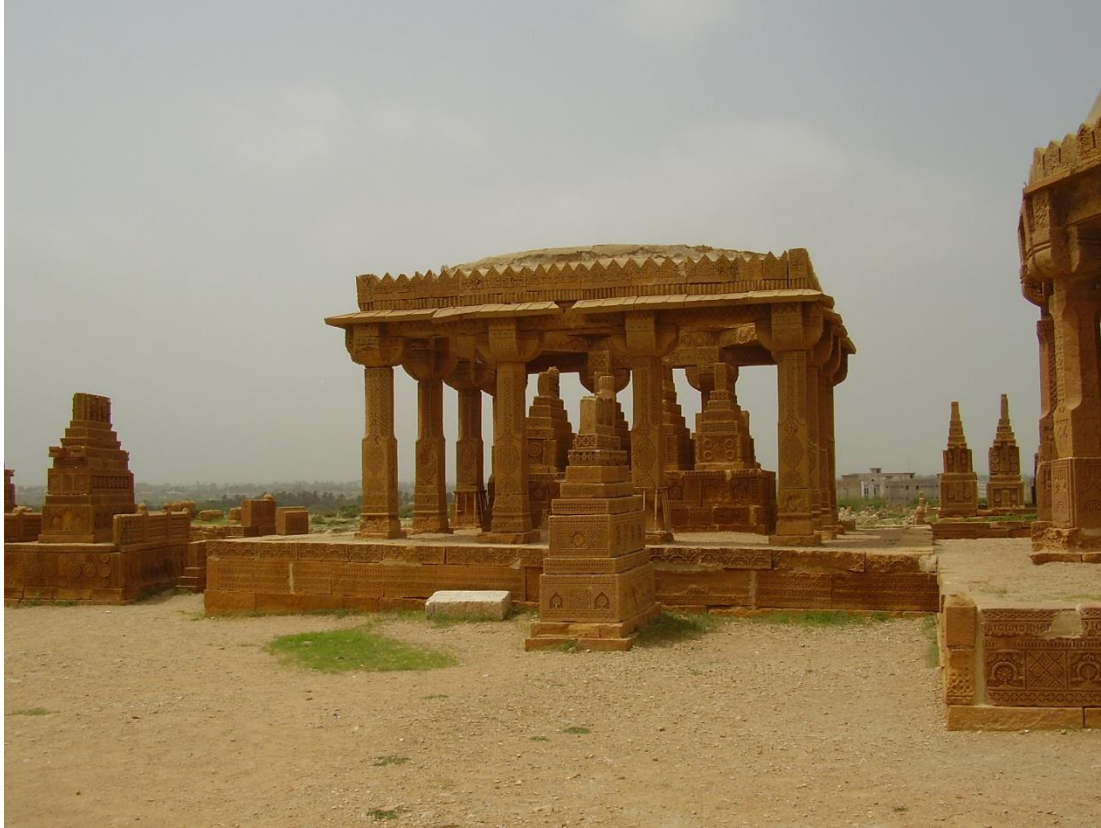
Fig 34. Showing a square canopy with broken dome.
