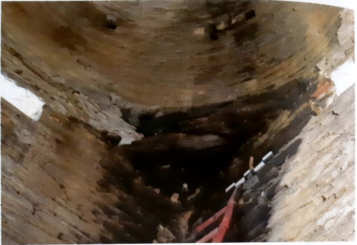
Fig. 63 - The three SE corner beams and S clerestory lintel (Photo by EL).
