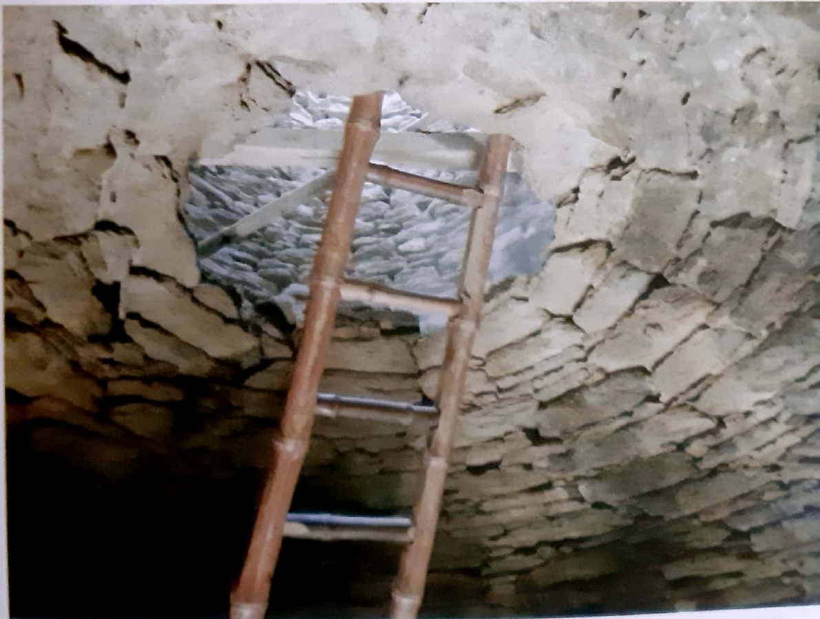
Figs 9-10 - Conservation in progress (below: a detail of the double domes) (Photos by FM).
