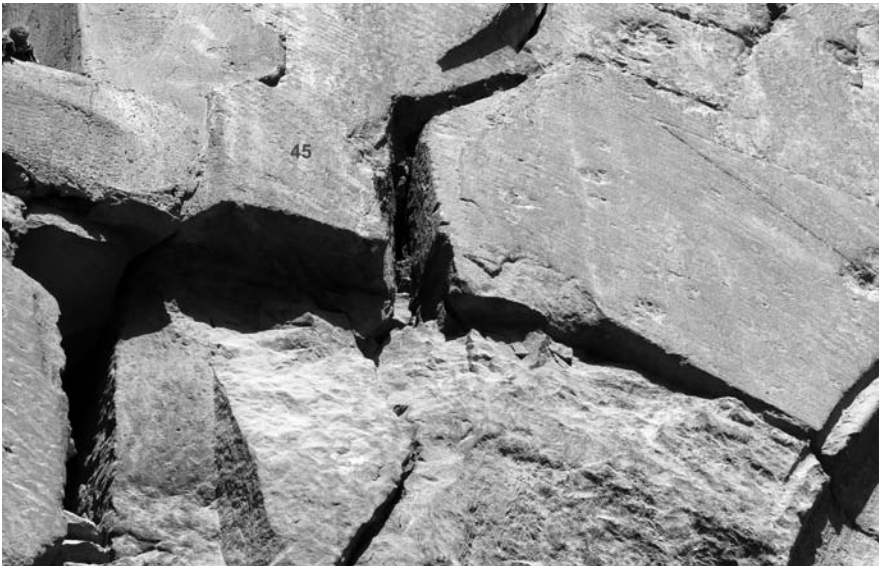
Figure 14.7 Eastern external wall; detail of the jamb of niche 8, US 45; see Figure 14.9 (photograph by C. Tonghini)
