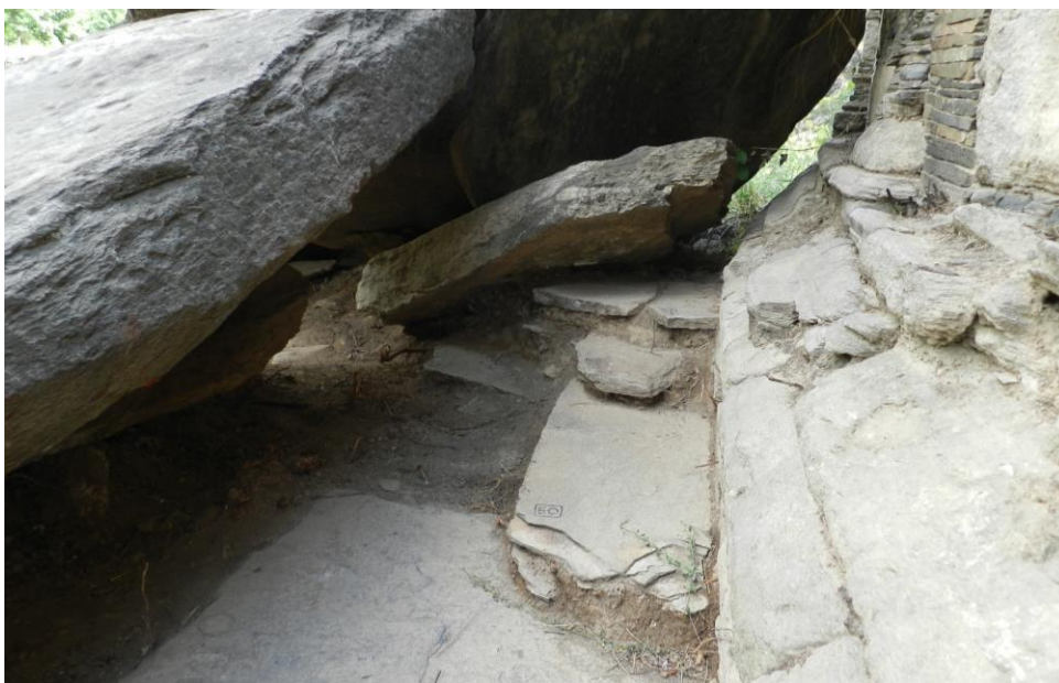
Figs. 30-31 - Two views of the chattras on the E side of the top floor of the podium. The picture above shows also the rows of brackets and coping that mark the upper storeys. In correspondence with the collapsed chattras, the row of brackets is missing. The left picture shows traces of four of the superimposing floors on the top of the 1st storey. (Photos by LMO).
