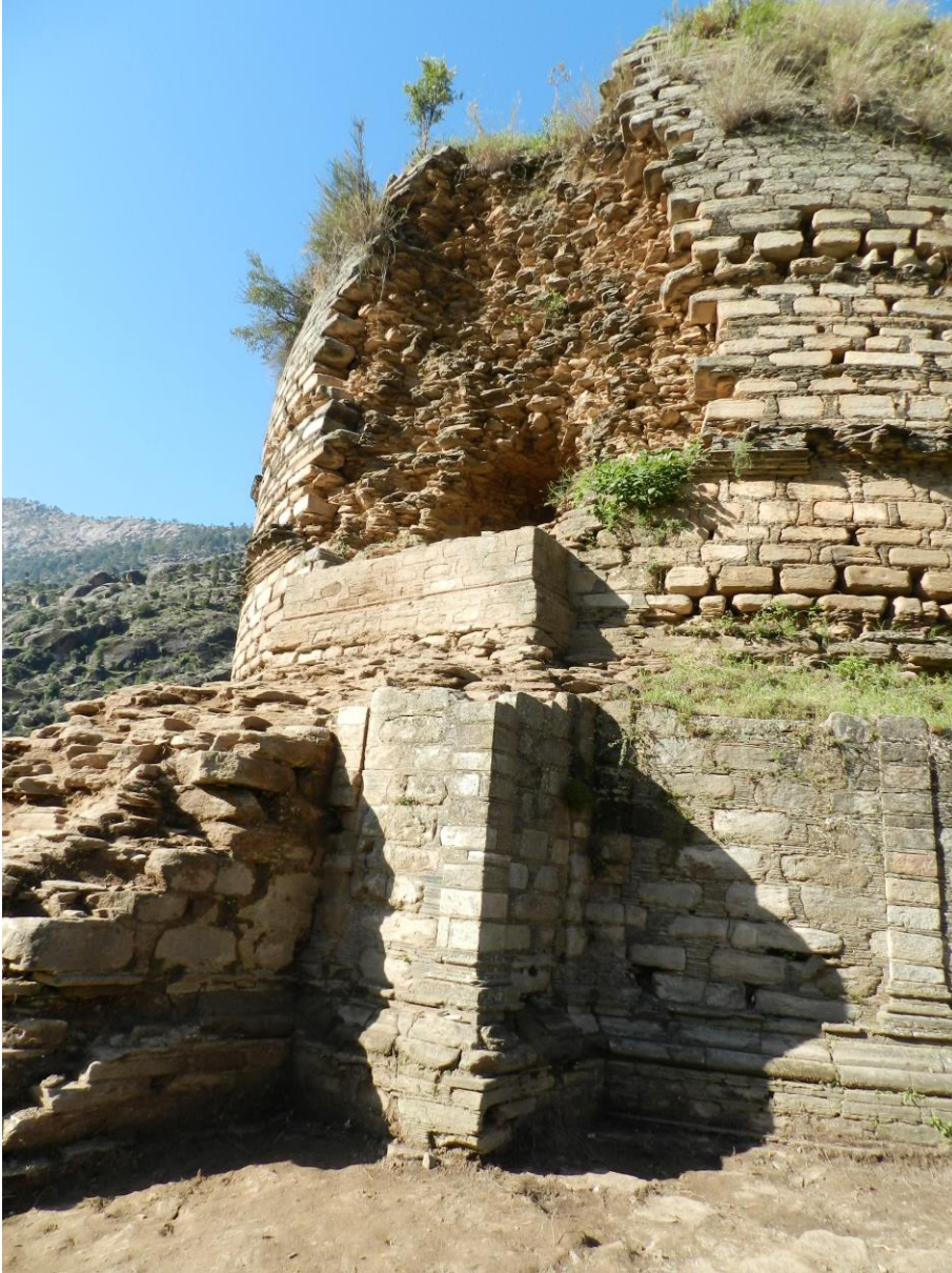
Figs. 28-29 - The 1st stairway (left); the 2nd storey, the 2nd stairway and the upper pediment. (Photos by LMO).
