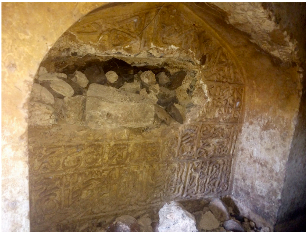
Figure 7. Funerary complex of the Bahmani dynasty. Tombstone in the north-western niche with a large crack in the upper part. Ashtur, India (photo: S. Mondini, 2015)
