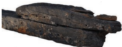
Fig. 4.7. Detail of the joint between floor timber 1 (corba) and its futtock (forcame) (photo: C. Beltrame)
