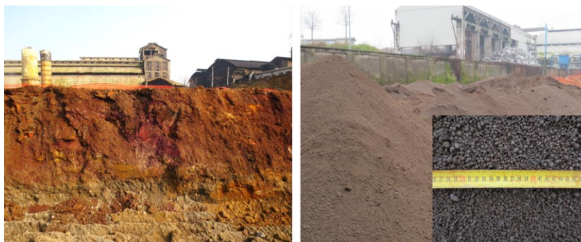
Pictures of the excavation front with pyrite ashes (left) and the granulates after treatment (right).
