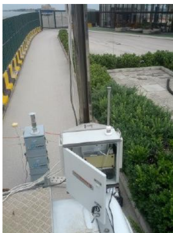
Figure 2.25. The OPC installed in Brindisi site in 2014.
