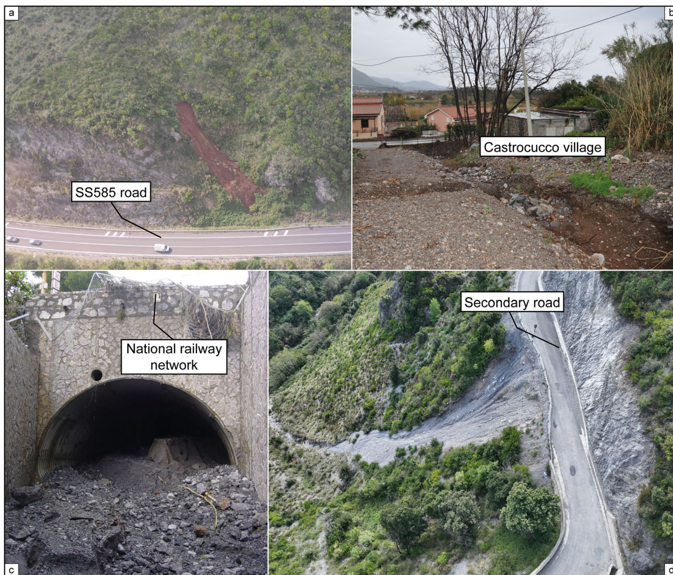
Fig. 12 Photo collection of damages at the urban area and infrastructure of the October 2022 event, with the landslide affecting (a) the national road SS585, (b) the urban area of Castrocucco, (c) the national railway network in Marina di Maratea, and (d) a secondary road
