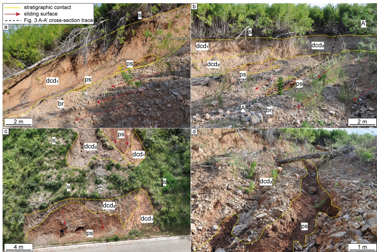
Fig. 2 Examples of crown areas used to reconstruct the stratigraphic succession, individuate the sliding surface, and sample the investigated levels (br: ancient cemented breccias, ps: paleosoil, dcd 1 : finer detrital and colluvial deposits, dcd 2 : coarser detrital and colluvial deposits, s: soil)
