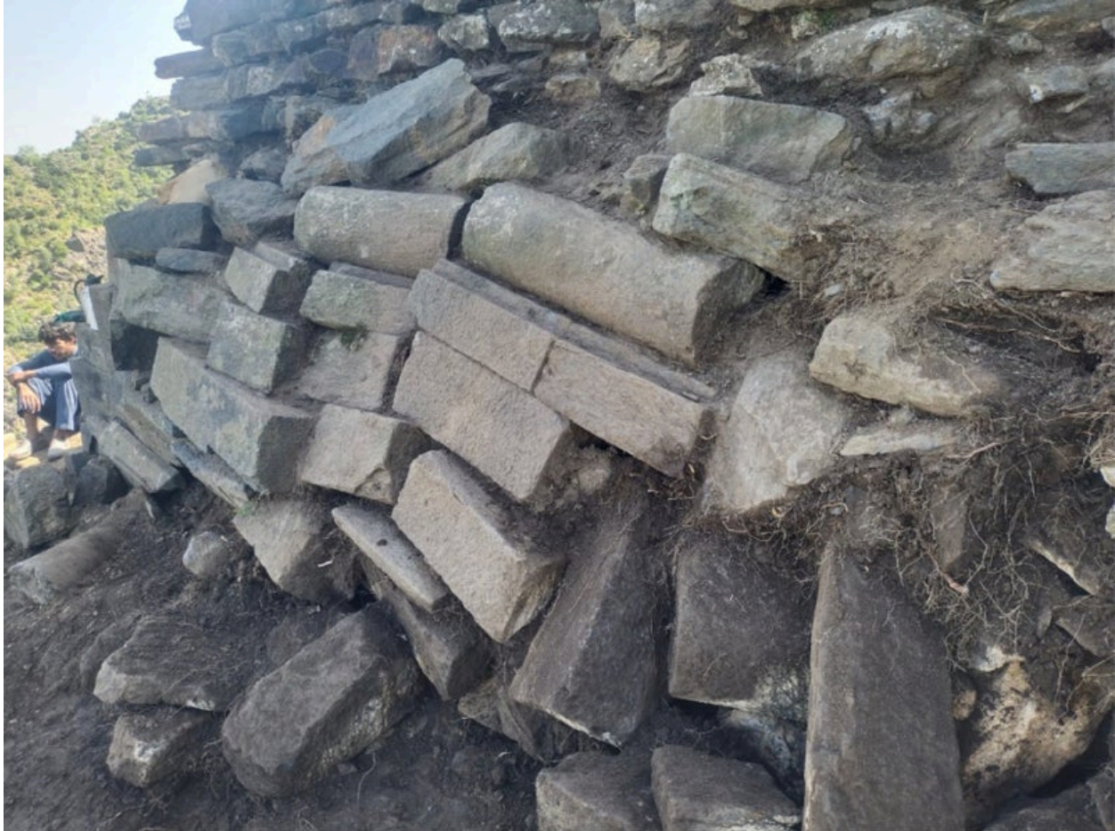
Fig. 93. Trench HDZ I: Traces of displacement at the bottom of the northeast corner of the upper podium (Khyber PATH, CC BY-NC-ND 4.0)
