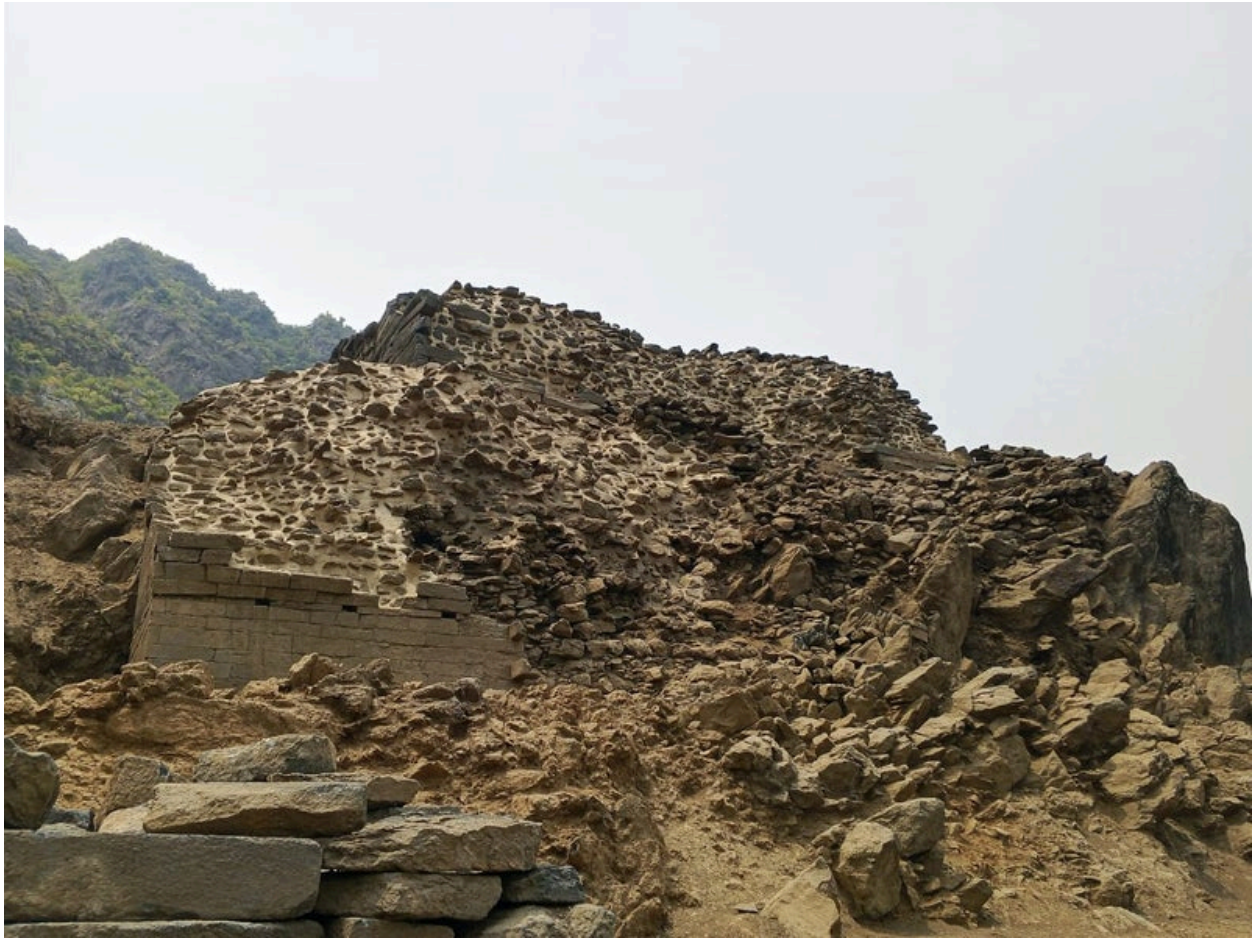
Fig. 91a–c. View of the east side with the ruined stairway during the conservation activity, May 2026 (Khyber PATH, CC BY-NC-ND 4.0)
