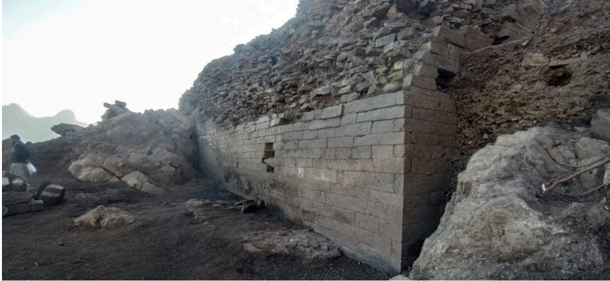
Fig. 92. Trench HDZ I-1: The lower podium of the “Takht” at the end of the operation (a view from west-northwest) (Khyber PATH, CC BY-NC-ND 4.0)
