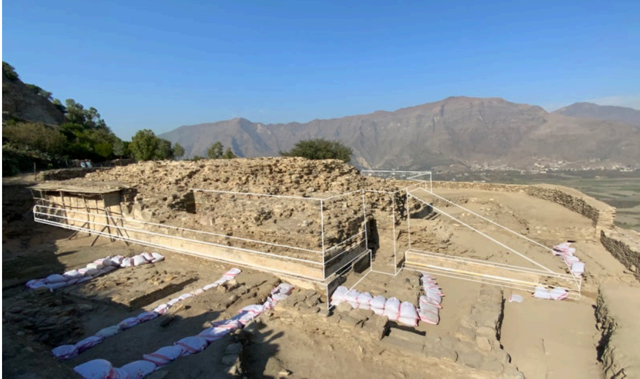
Fig. 53. Restoration of the elevation of the podium of Temple 6 in Period 2b (Alice Casalini/IAMP, CC BY-NC-ND 4.0)
