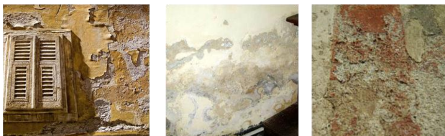
Figure 1. 4 examples of damage caused by water action and moisture on mortars, from left to right: detachments, spots and bio-fouling, powdering
