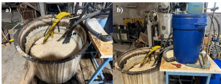
Figure 6.2: Nitrification (a) and denitrification (b) tanks.
