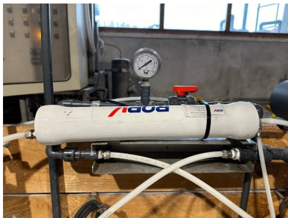
Figure 6.5: Reverse osmosis membrane
