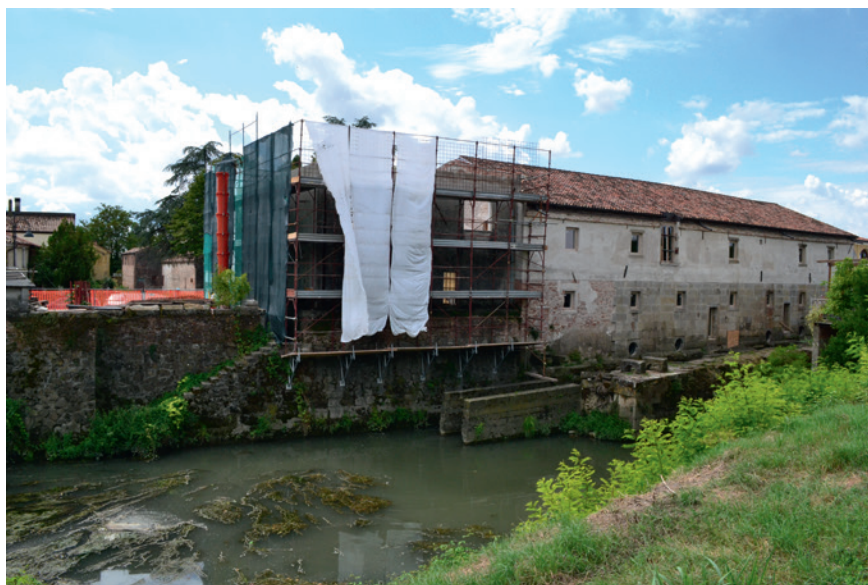
FIGURE 8.4 Recovering seventeenth century water mill, with stone steps leading to mooring dock
